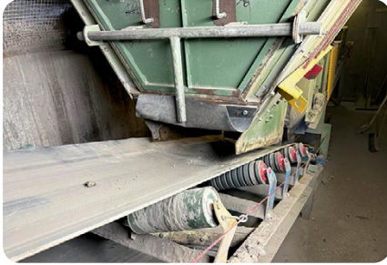
Before installation: excessive dust and spillage increased clean-up efforts and reduced overall.
