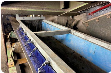
Transfer Point with installed AirScrape® and K-Containment® Seal.
