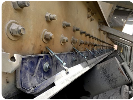
Mining company in Peru has equipped seven conveyors with AirScrape and plans to expand the installation to other conveyors.
