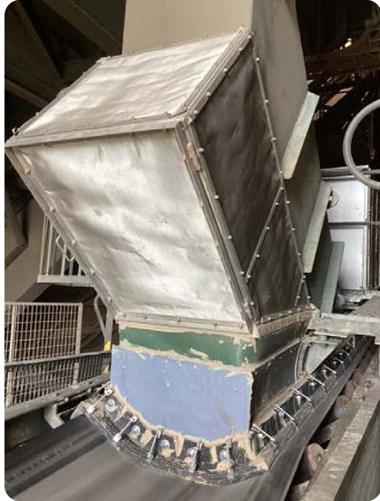
The excess dust has been successfully contained and soiling has now been reduced to zero.
